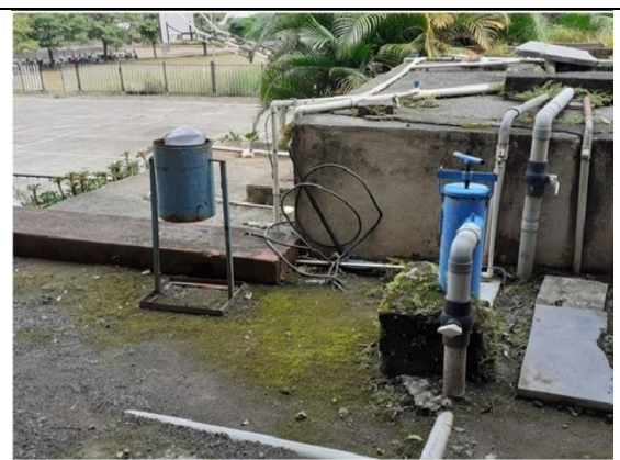
Rainwater Harvesting ( Storage Tank)
