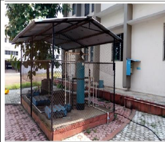
On campus sewage Treatment Plant
