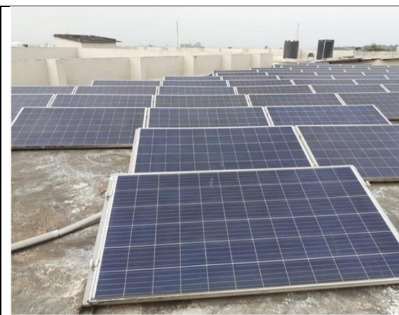
Roof top Solar Panel
