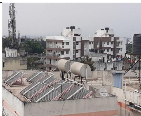
Solar Water Heater
