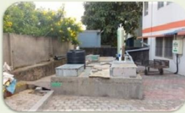
Sewage Treatment Plant (Location: Girl Hostel)
