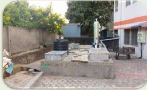
Sewage Treatment Plant (Location: Girl Hostel)
