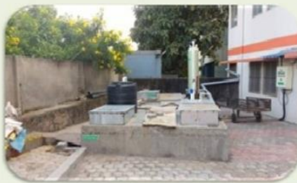
Sewage Treatment Plant (Location: Girl Hostel)
