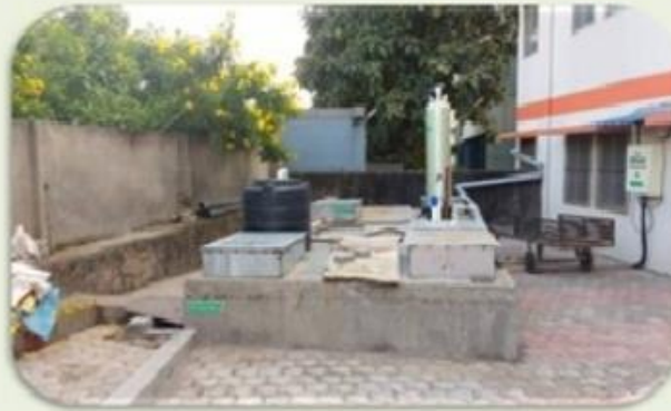
Sewage Treatment Plant (Location: Girl Hostel)
